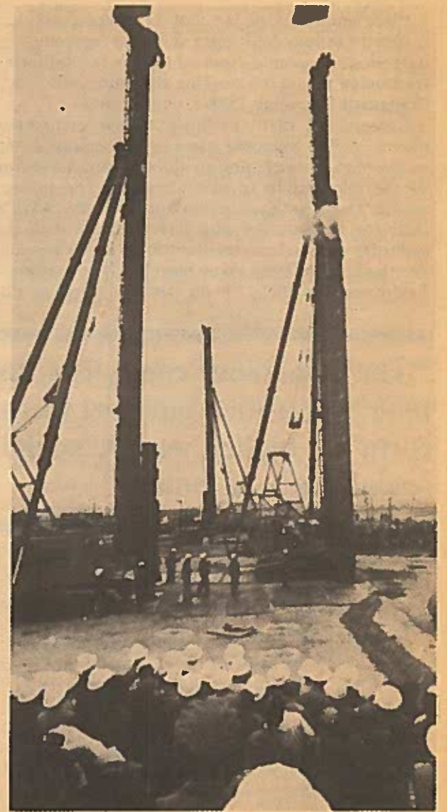
The first pile is driven for a new steel mill in Shanghai, one of the many industrial plants that are being built in China with the help of American, British, Japanese and West German corporations. Each plant is "purchased," with a multi-million dollar loan from a group of western imperialist banks. When this mill is running, the Chinese bourgeoisie will share the profits produced here with those bankers.
