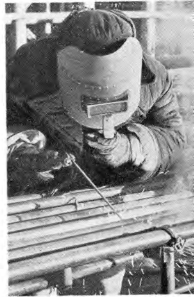
Two women welders on the construction site of the Taiyuan Power and Heat Plant
