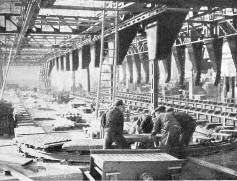
Workers completing installations in the foundry of the State-owned Chingwei Textile Machinery Works in North China, the first up-to-date works of their kind in China. They finished their work 10 days ahead of schedule
